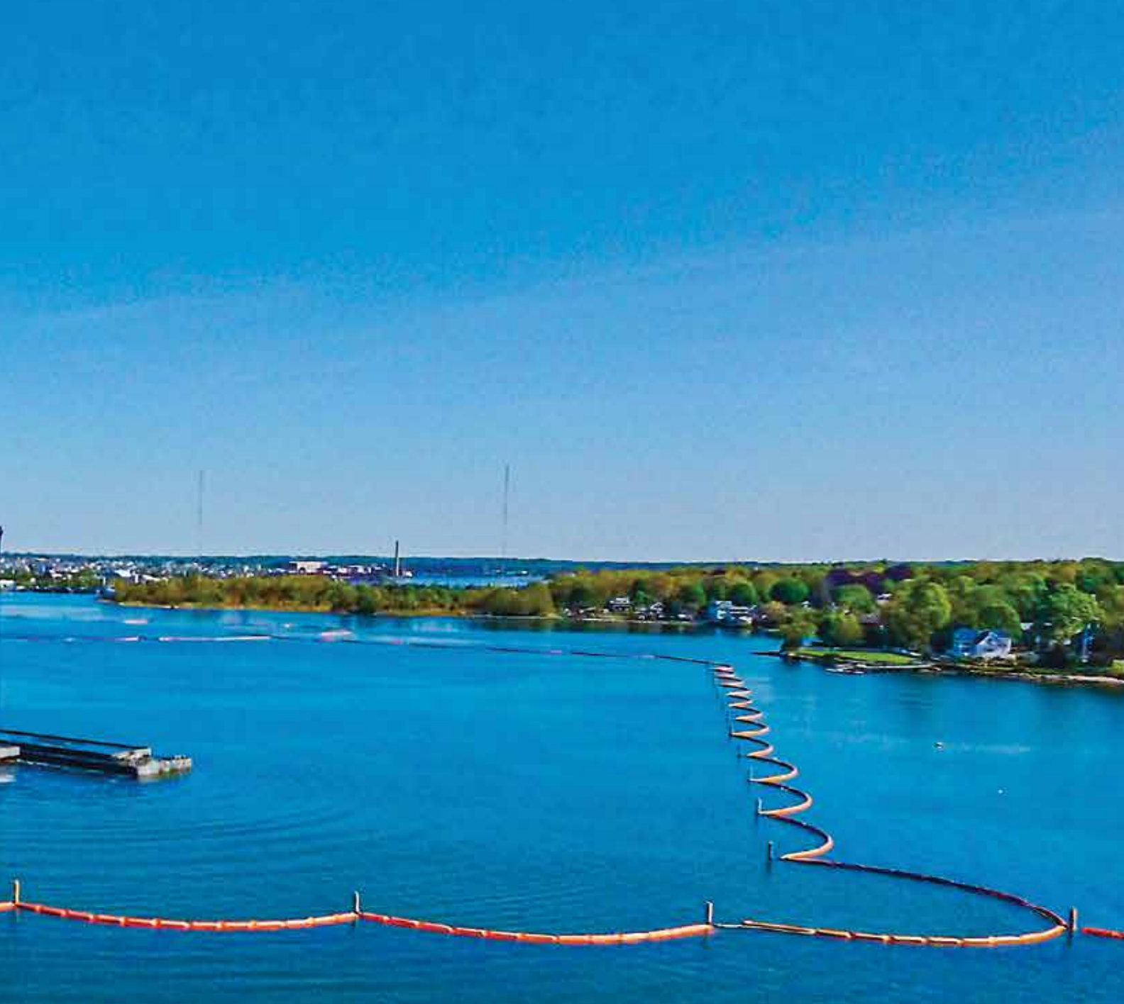
Figure 1: New Bedford Cell Construction Credit - “Foth Infrastructure & Environment, LLC” Cashman Dredging & Marine Contracting Company, LLC - Dredge AJ Fournier - Scow Joe Verrochi; AGM Marine Contractors, Inc Dredge - Triton - Scow 1501; Cashman Dredging & Marine Contracting Company, LLC - Dredge Wood 1 – Scow Patriot 144, Wood 1 and Triton are dredging in Top of CAD 4. AJ Fournier dredging in Middle of CAD/CAD 4 Access Channel.
