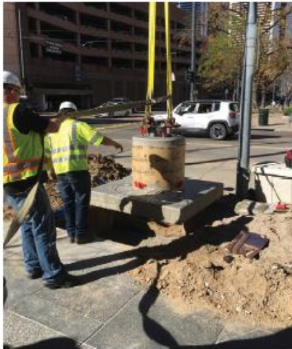
Step 1: Place pre-cast foundation and grounding into excavation in the right-of-way. (Caisson optional.)
