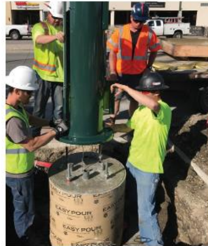
Step 2: Install base cabinet of the CityPole® onto the foundation and secure
