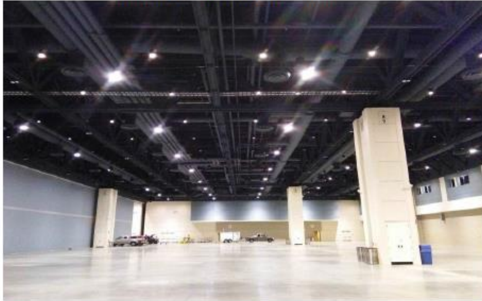
Graybar Brings Great Lighting and Energy Savings to the Raleigh Convention Center
