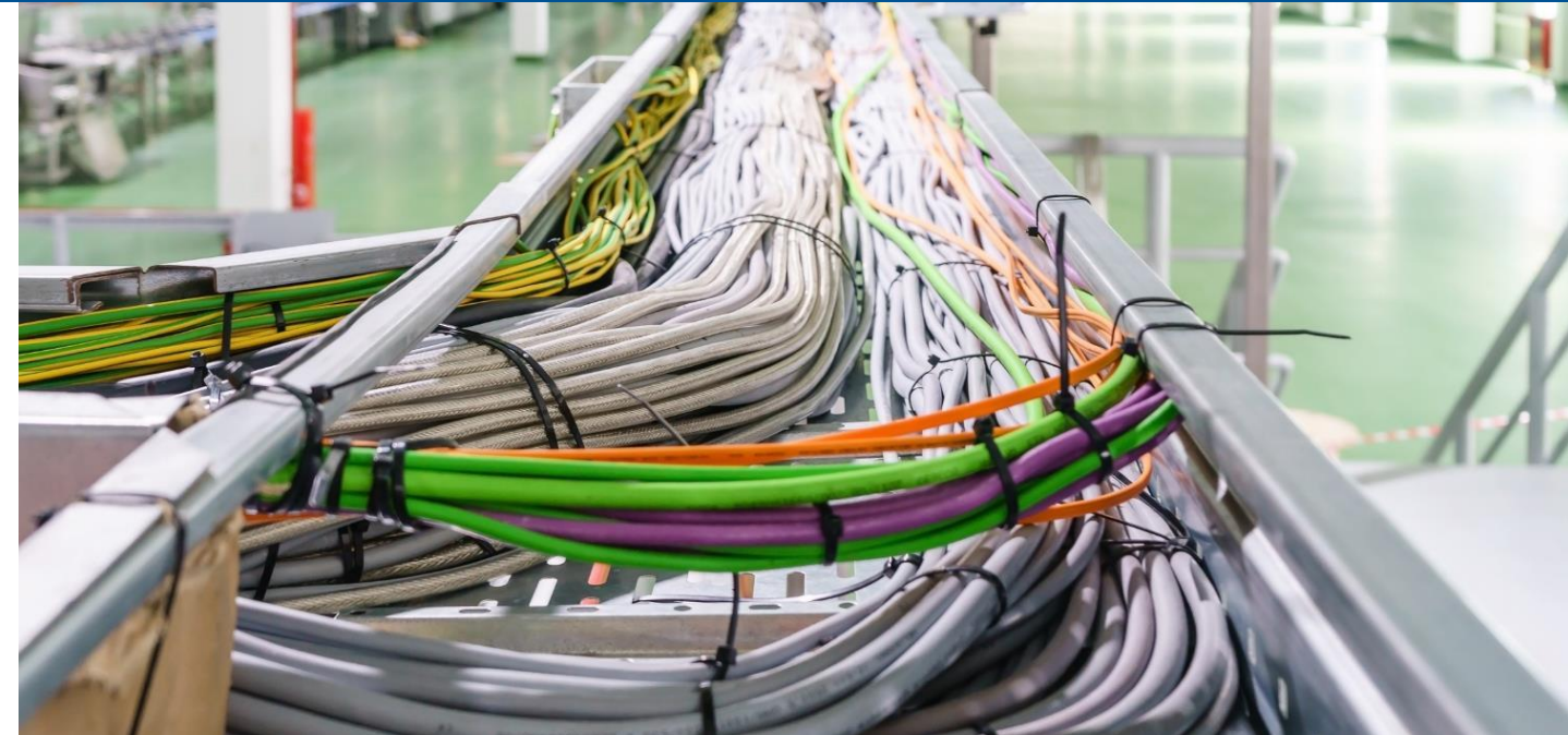
Multiple layers of single-purpose infrastructure
