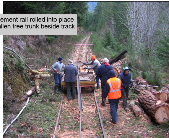
Crew lifts replacement rail onto car at Loon Lake. Note 'Hi-railer' behind.
