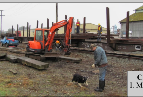
Unloading Rails Bee - January 29, 2011 (l.) R. Catto operates crane truck while Big Steve steadies the load. (below) J. Jansma being trained by Sam while K. Fyfe moves concrete slabs into place.
