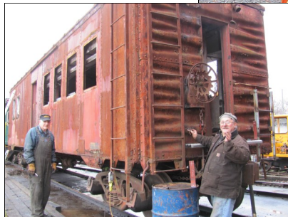
Upgrading boxcar Rollie Hurst (l.) and Dan Gledhill work on the boxcar to be used in BCIT Conductor training, bringing it up to modern standards.
