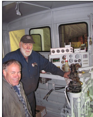
Re-installing the controls & wiring in cab Sterling Stump (front) & K.G. Campbell Photos: D. Hooper
