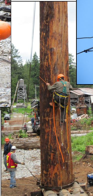
(right) Gerard on the way up the tree. Note the McLean Mill water tower in the background and the abutments for the bridge across the new Creek channel.
