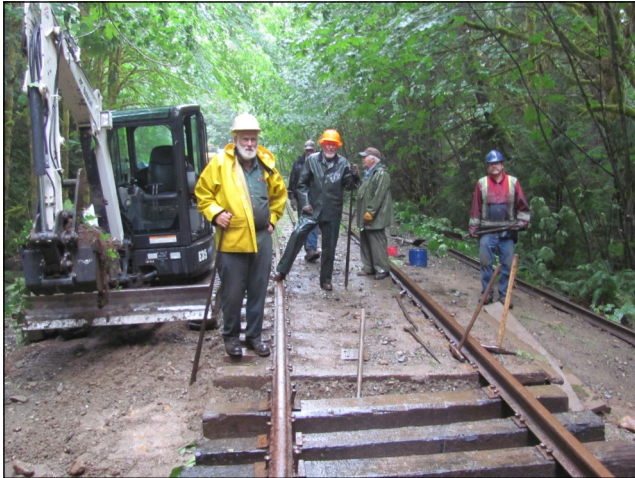
(l.) Track Repair near Bainbridge Ken Fyfe's excavator is beside the repaired track. The machine simplified the job immensely. The 'Hi-railer' and the 'A-6' speeder transported the crew and the excavator on its rail car out to the site. (l. to r.) Soup Campbell, Harold Carlson, Ken Fyfe, Don Wigen.
