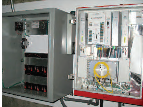
Power backup unit with SOLiD ALLIANCE remote.
